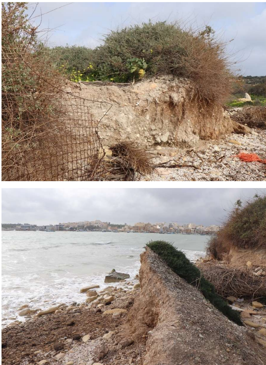
Figure 14 – A section of the perimeter of the saline marshland showing impacts arising from wave action and potentially leading to coastal erosion.
