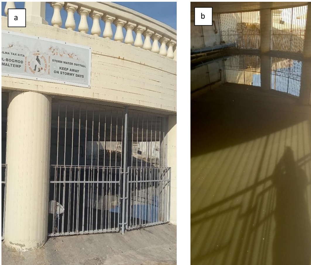
Figure 16 (a,b) Ta' Xbiex Stormwater Outfall
